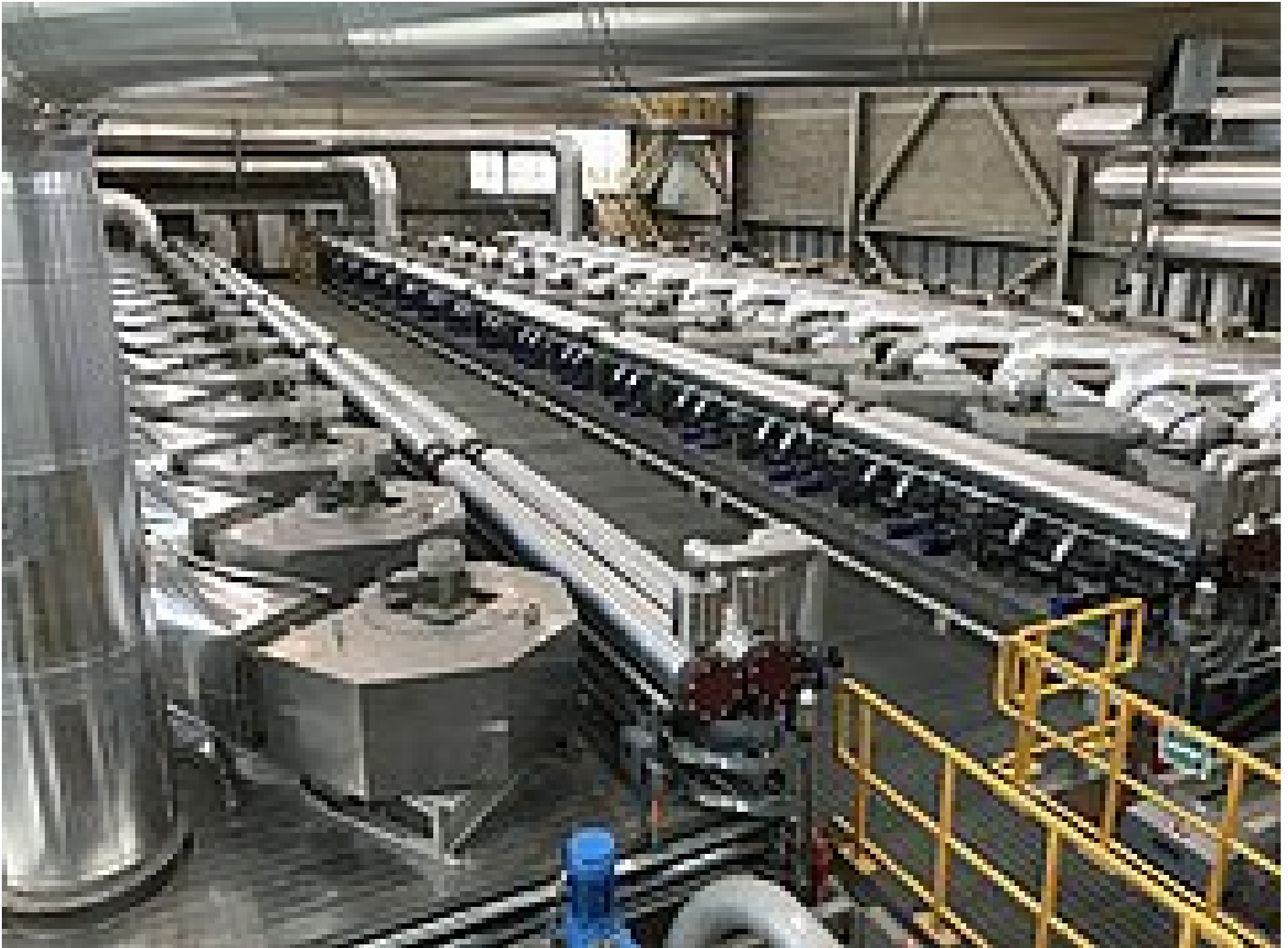
Impressive size: Three HUBER Belt Dryers BT 30 at new Bello wastewater treatment plant
