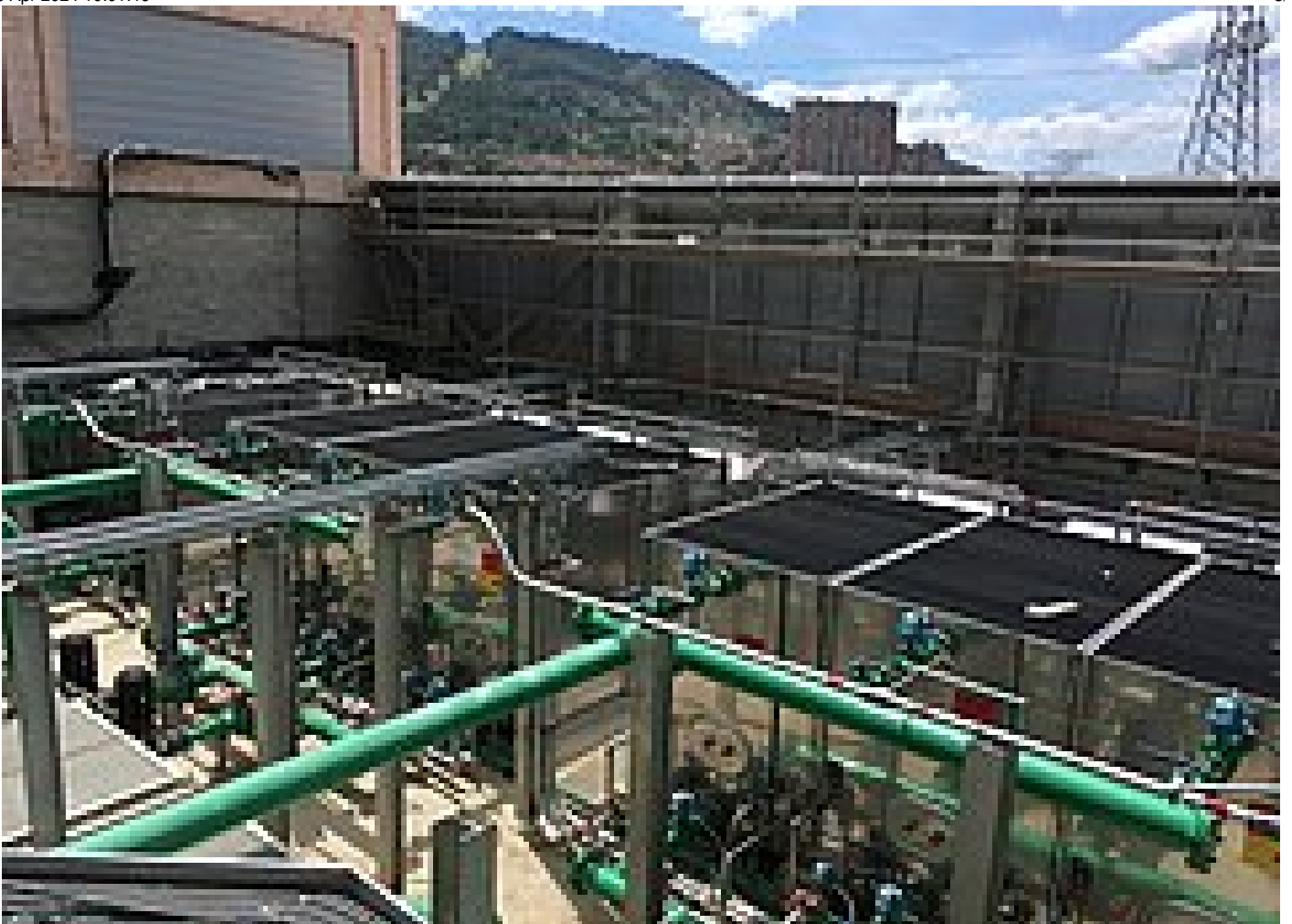
Cooling towers and exhaust air treatment
