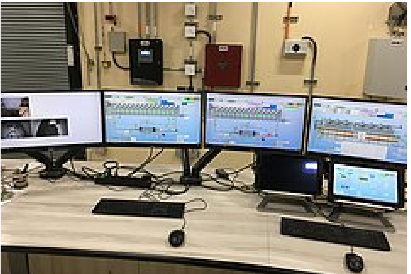
Control system for the drying plant
