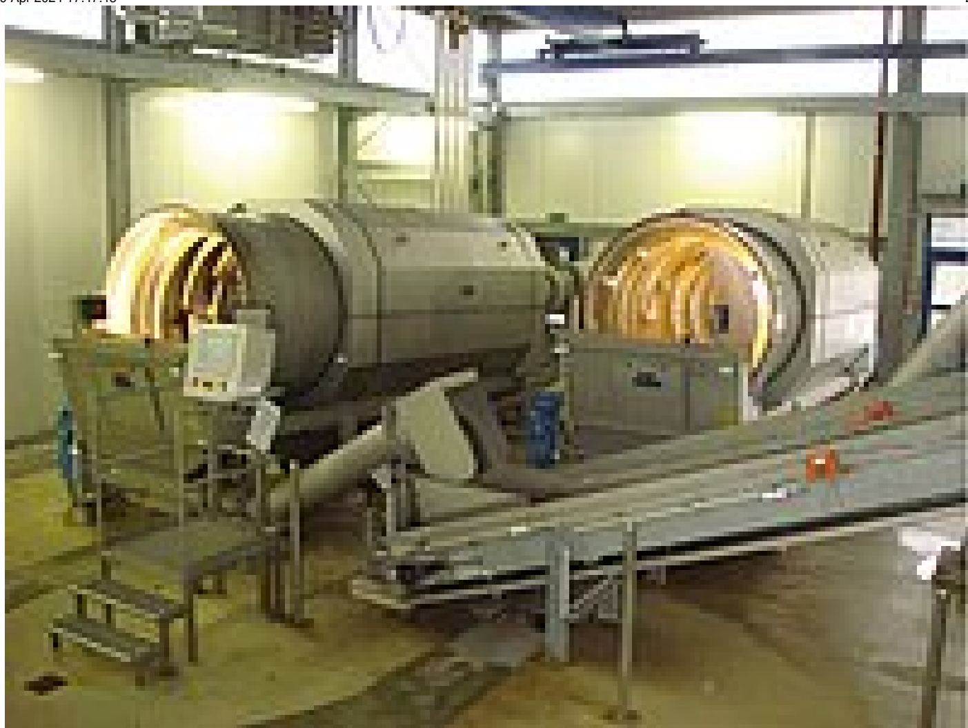
Two ROSF 9 wash drums with WAP screenings presses for the removed and washed coarse solids
