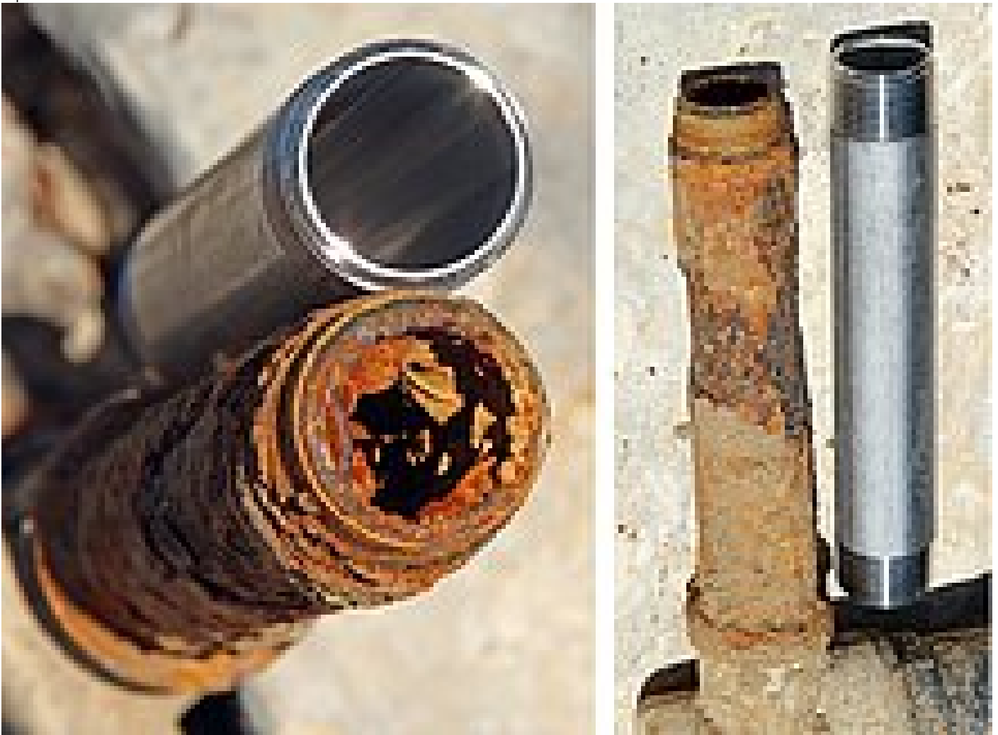
Figure 5. Extreme example of corrosion of a galvanized steel pipe after 6/7 years in a water supply system (TX, USA), compared to a stainless steel pipe (Raines, 2018)
