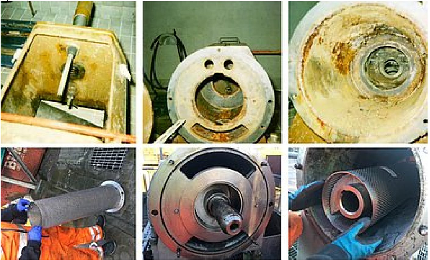
Figure 6. A comparison of various components of two similar sludge screens. The pictures above reveal components of a coated carbon steel screen with extensive corrosion after 12 years. The pictures below reveal components of a stainless steel screen after 12-13 years with no corrosion.
