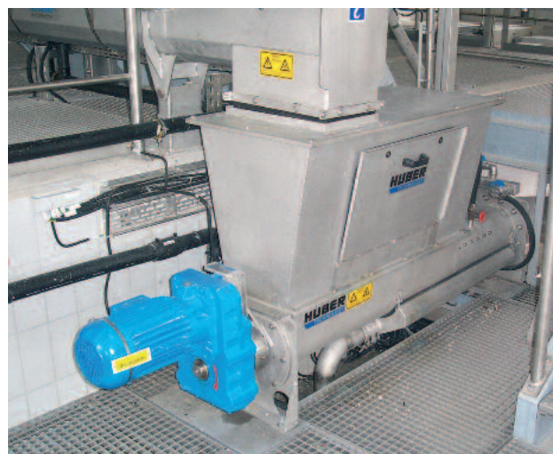
WAP with a large hopper, fed via a screw conveyor
