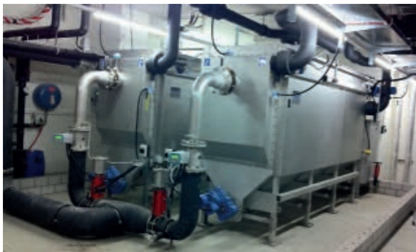
RoWin Heat Exchanger size 8 installed in the second basement of the Wintower building at Winterthur
