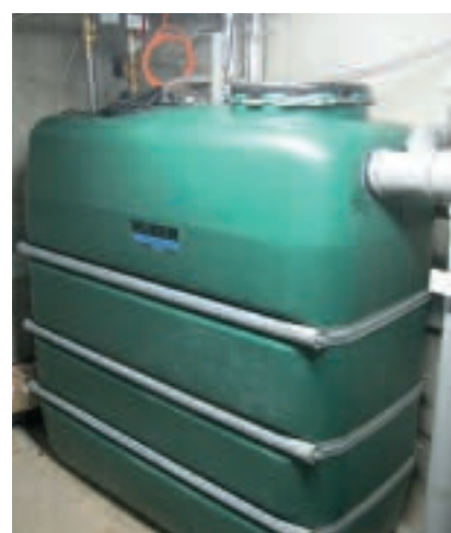
HUBER greywater recycling plant installed in the basement of the hotel, and technical data
