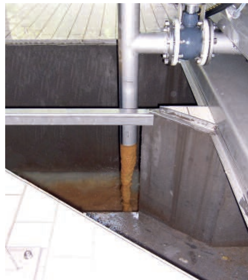
The wash water with its high carbon load is returned to improve denitrification and gas yield
