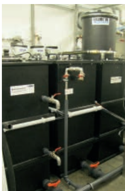
Picture 2: MBR greywater treatment plant
