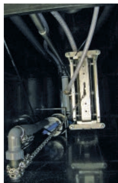
Picture 3: Membrane ultrafiltration unit
