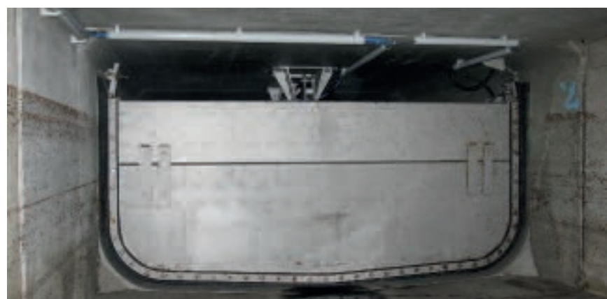
Flushing gate installed in a rectangular storage sewer
