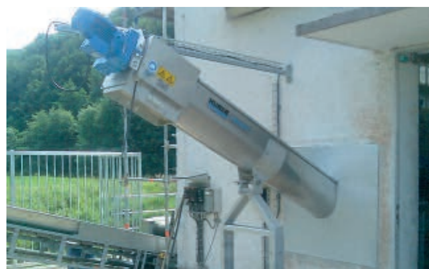
Automated screenings removal
