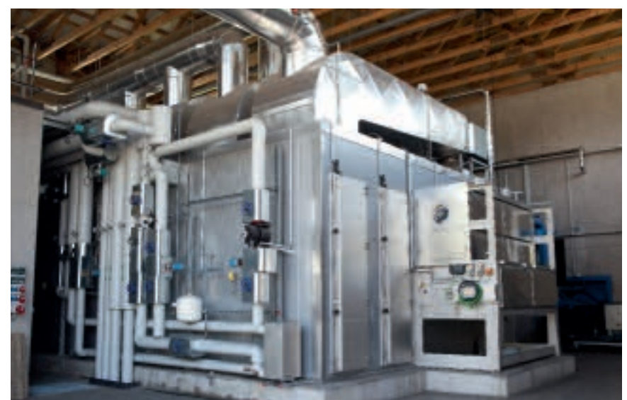
Belt dryer on WWTP Balingen with two temperature zones for efficient sewage sludge drying
