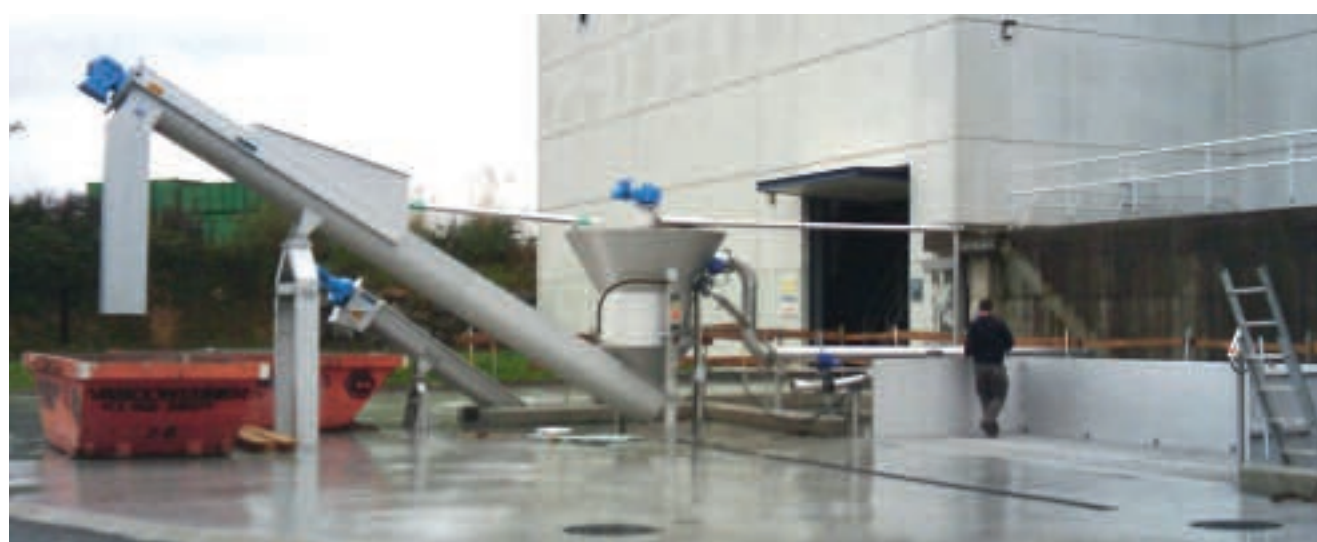
The acceptance area of the sewer grit treatment plant at San Sebastián
