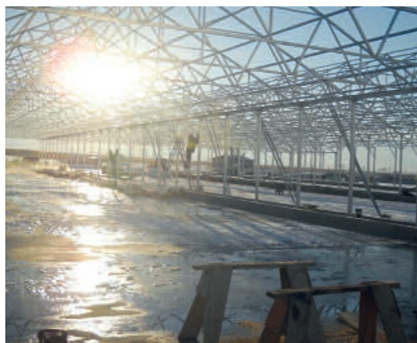
Solar dryer under construction at Utah – a reasonable solution even in climate zones with cold winters
