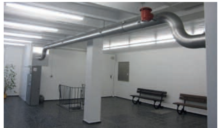
Air line with safety valve
