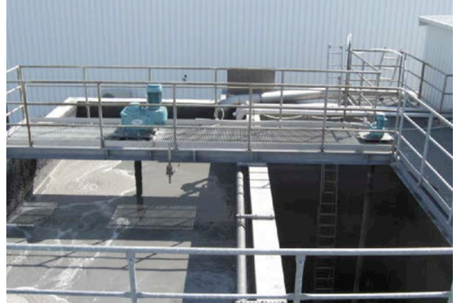
Biotank (left), mixing & balancing tank (right)
