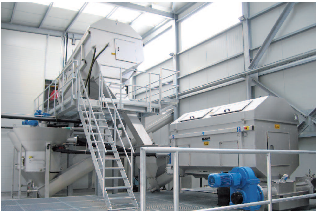
HUBER Wash Drum RoSF 9 with two subsequent HUBER Grit Washer RoSF 4 units, coarse material washer, ROTAMAT® Rotary Mesh Screen RoMesh® for organics removal and compaction
