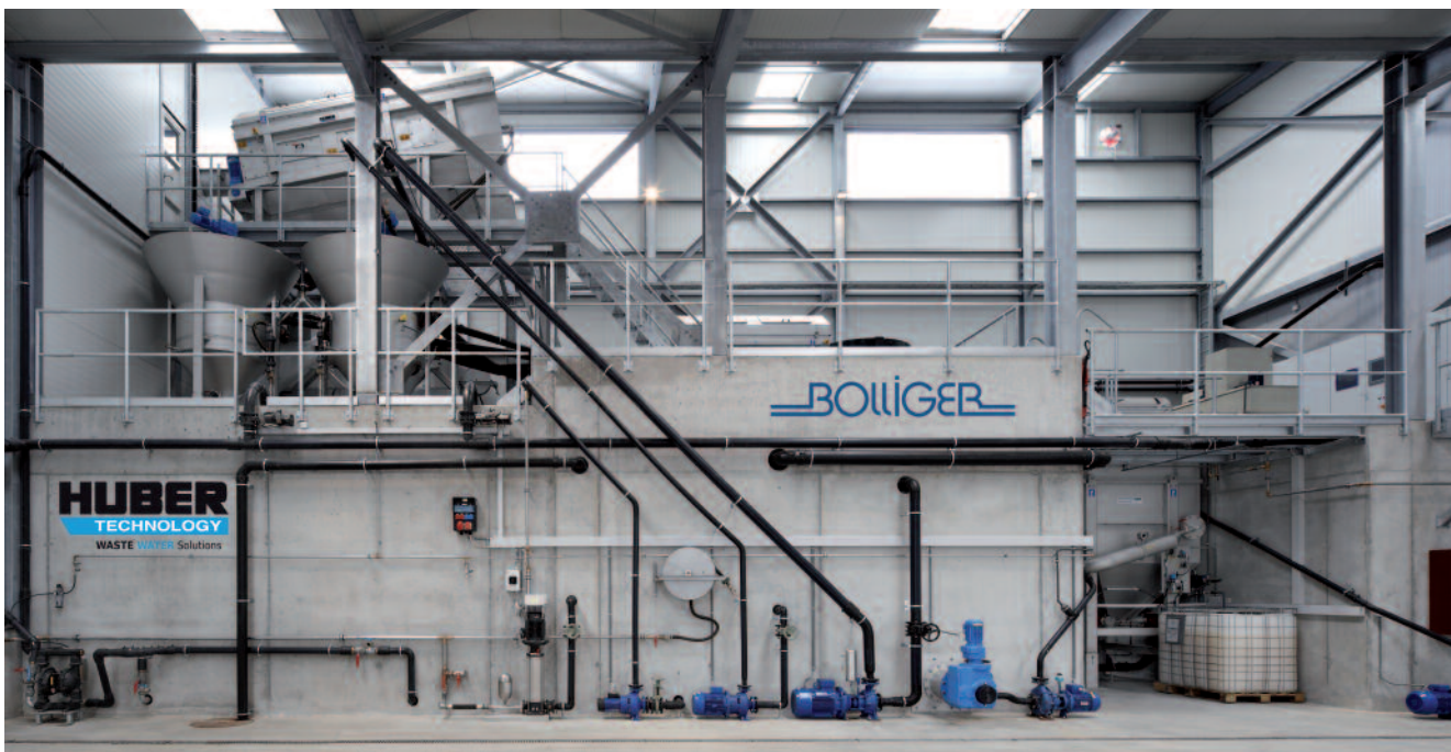
Smart pump technology arrangement to ensure easy access for maintenance
