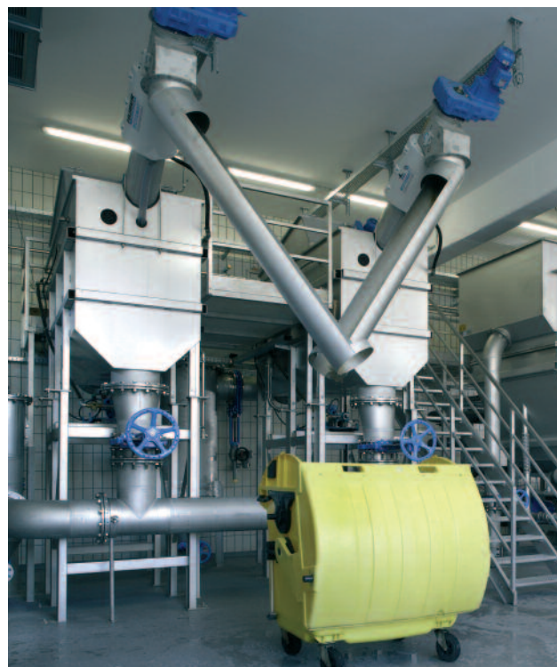
ROTAMAT ® Rotary Drum Fine Screen Ro 2 installed next to the HUBER Dissolved Air Flotation Plant HDF
