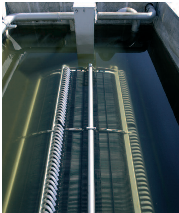
Flooding of the HUBER VRM ® membrane plant
