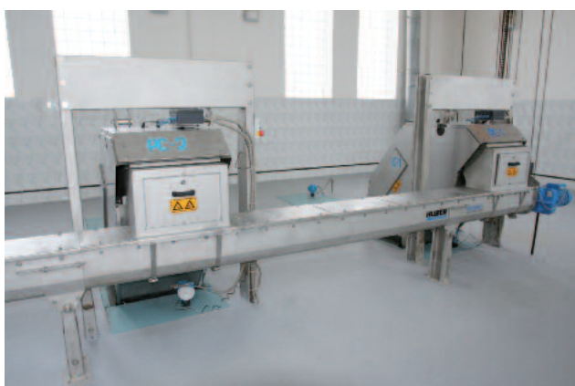
Two screens installed in parallel discharging into one screw conveyor
