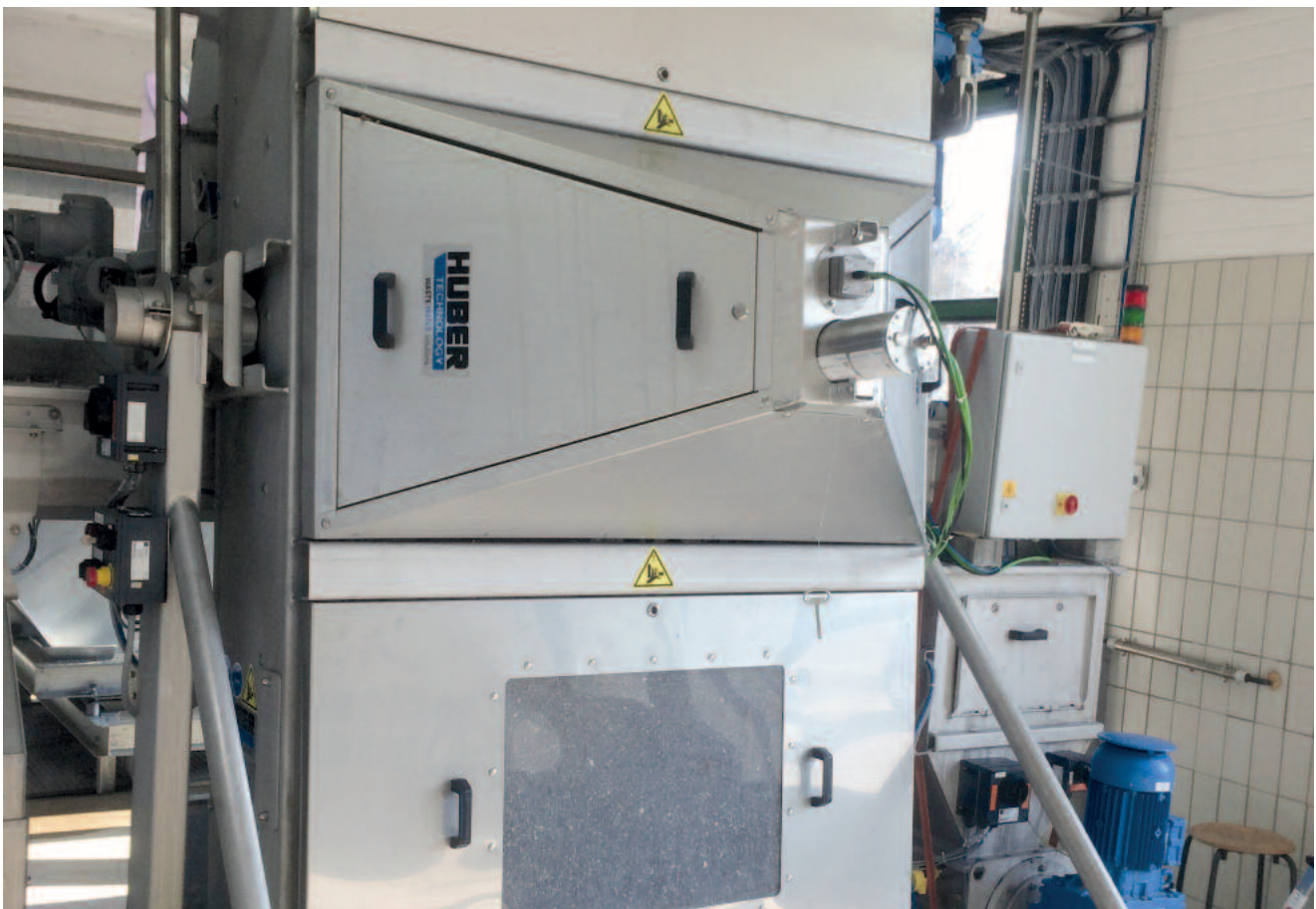
Fig. 1: HUBER Safety Vision system installed on a HUBER Multi-Rake Bar Screen RakeMax®
