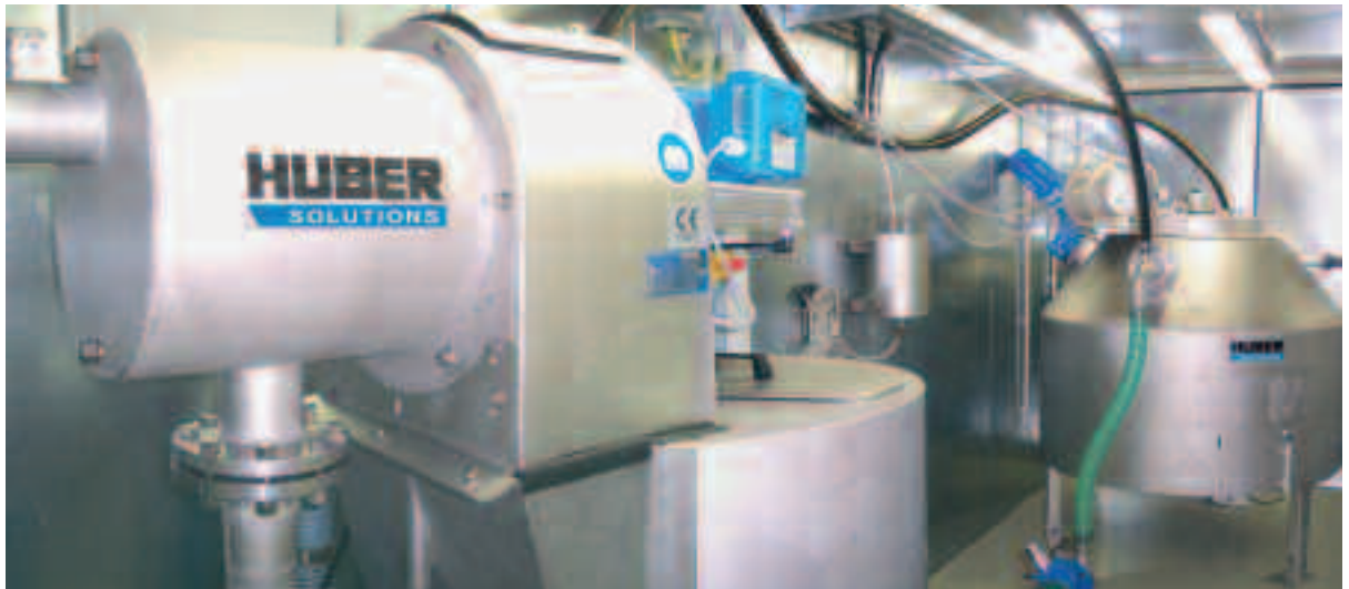
Anaerobic reactor for the digestion of black or brown water
