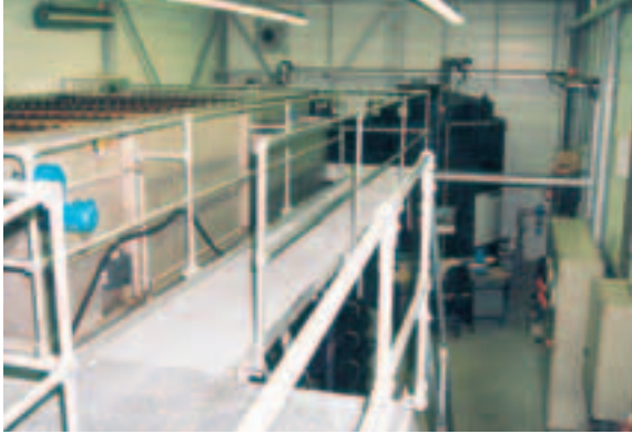
Slaughterhouse Hinwil / Switzerland, ROTAMAT® Wedge Section Screen Ro 2, HUBER Dissolved Air Flotation Plant HDF-50 with chemical treatment, throughput: 220 to 265 GPM (50 - 60m 3 /h), ROTAMAT® Screw Press RoS 3, throughput: 22 GPM (5 m 3 /h)
