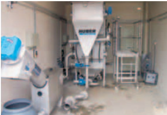
Butchery Walk / Germany: Meat processing ROTAMAT® Micro Strainer Ro 9 in tank, HUBER Dissolved Air Flotation Plant HDF-1 without chemical Treatment
