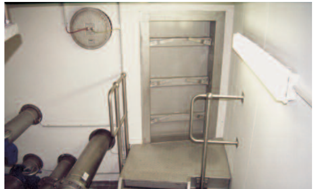
Access to water chamber
