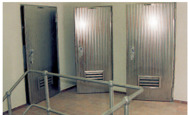
Hygienic, clean access area
