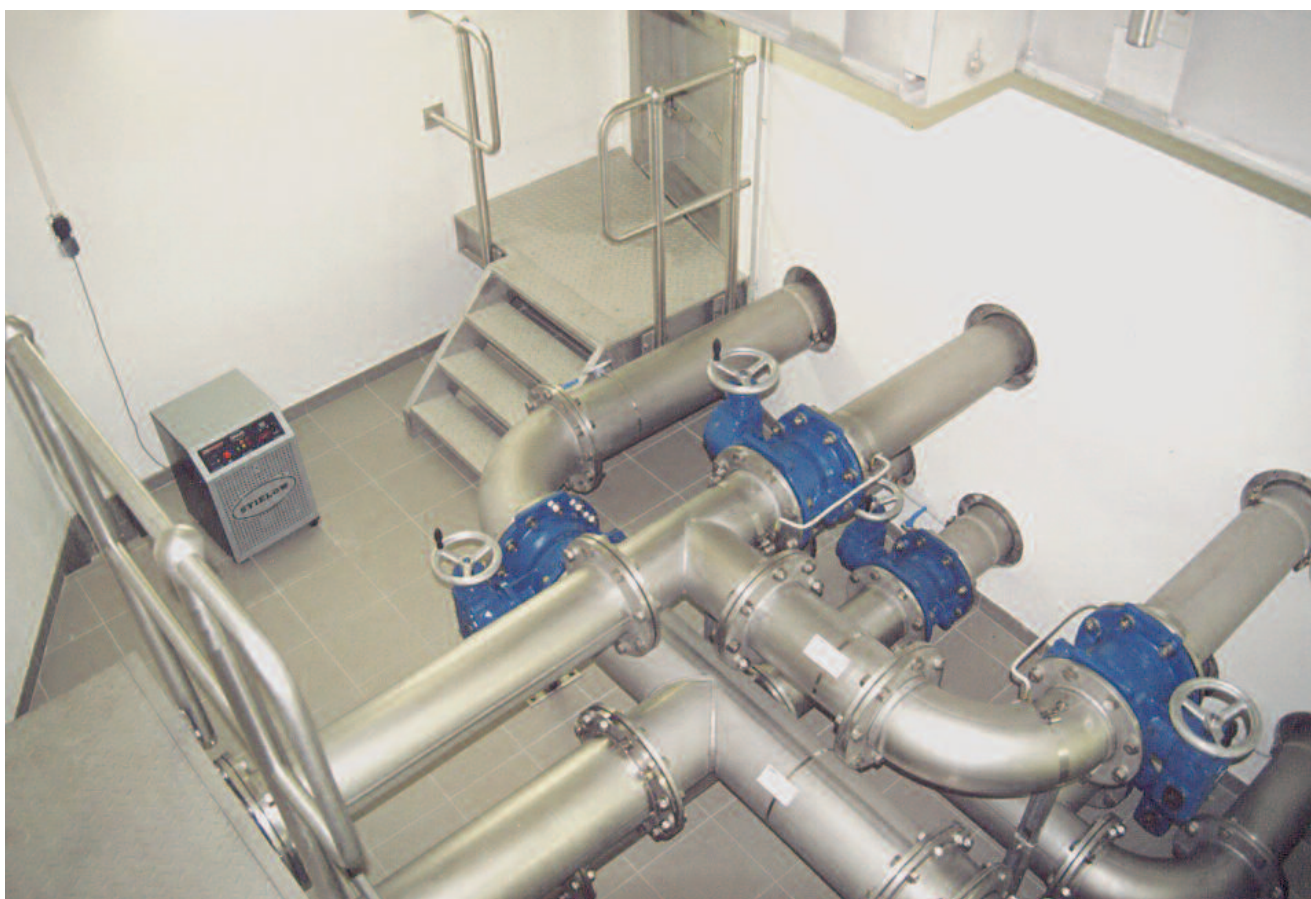
Clear pipework arrangement
