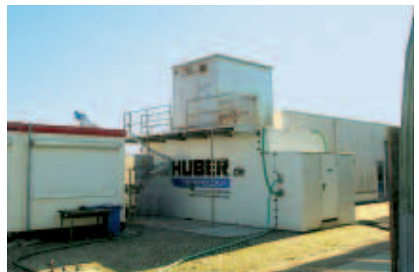
Membrane Bioreactor pilot-plant
