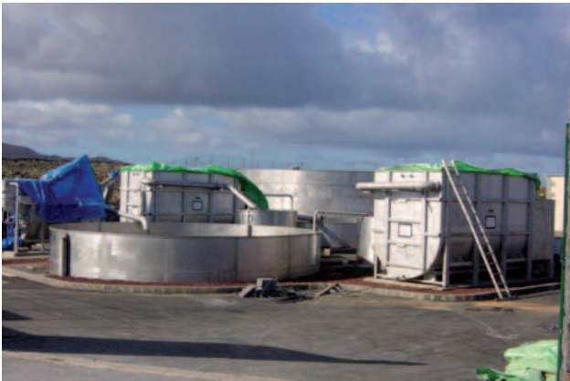
Two HUBER VRM® 20 units in tanks at the municipal WWTP La Santa, Lanzarote, Spain
