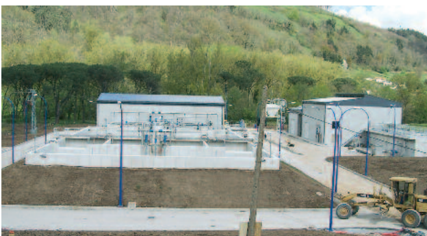
Four VRM® 30 units installed at the municipal WWTP Arenas de Iguña, Spain
