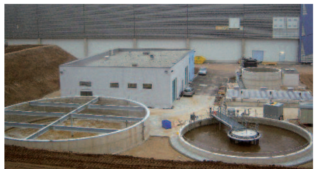
Three VRM® 30 units installed at the industrial WWTP Hans Kupfer & Sohn GmbH, Germany
