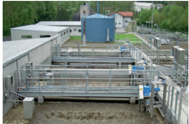
Three VRM® -units installed at municipal WWTP Hutthurm, Germany
