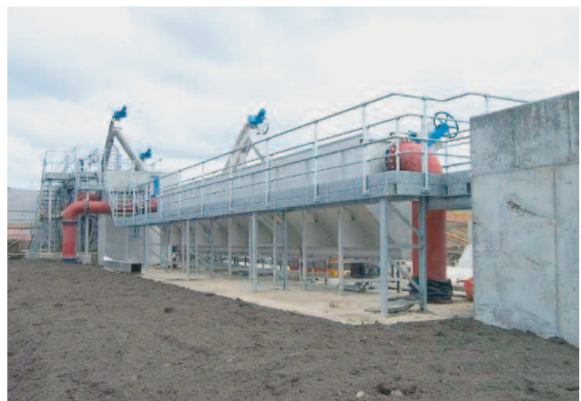
Above-ground installation of a ROTAMAT® Longitudinal Grit Trap Ro 6 with preceding screening
