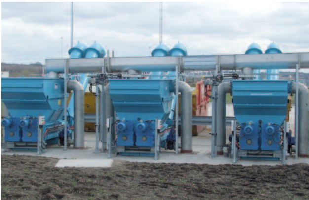
WWTP Knostrop (UK): 2 million PE HUBER Launder Channel: 20 m 3 wastewater per second
