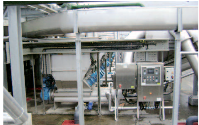
WWTP Dublin (UK): 2 million PE HUBER Launder Channel: 30 m 3 wastewater per second
