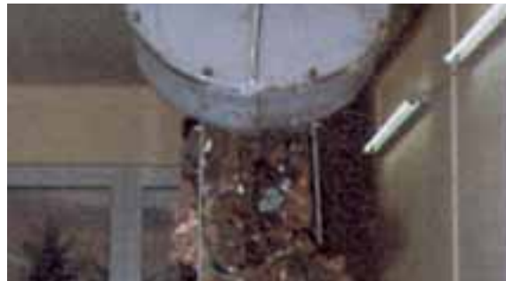
Discharge of screenings
