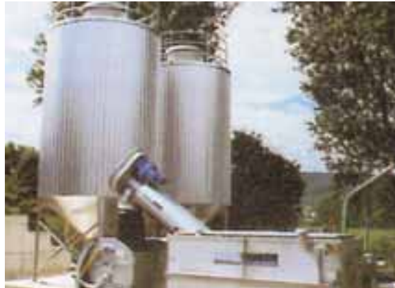
Thermally insulated balancing tanks permit continuous operation of the septic sludge treatment plant.
