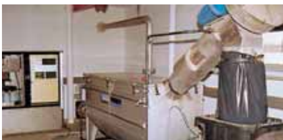
Sludge Acceptance Plant with metering, customer identification and automatic sampling.
