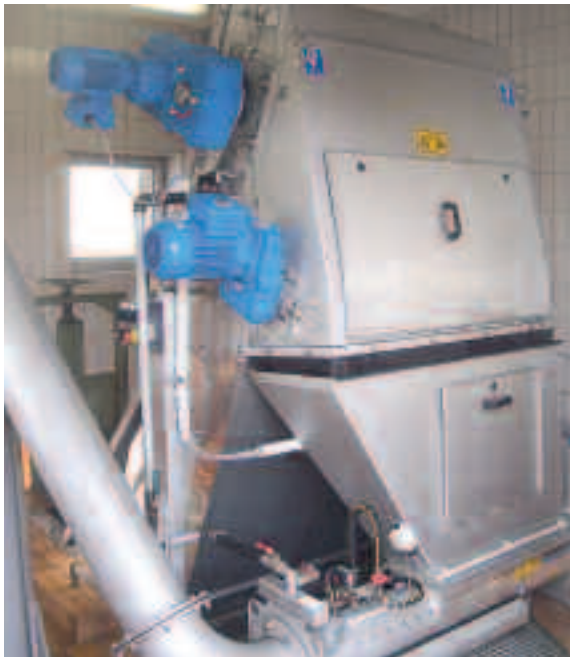
Rear view of the EscaMax® with subsequent Wash Press WAP
