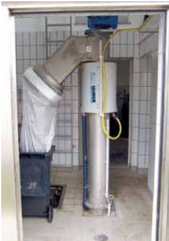
Screenings discharge into a bagger
