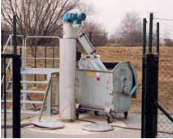
Thermally insulated and heat-traced unit
